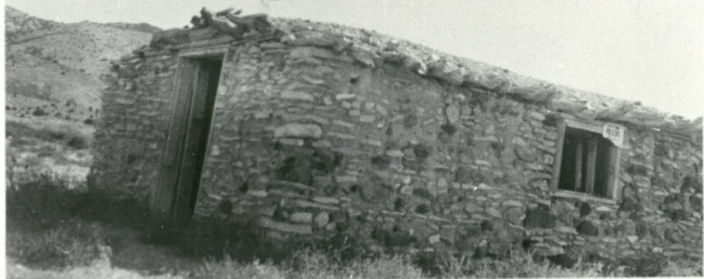
Old Rock stable at Simpson Springs. Regardless -- this is NOT the old Pony Express Stable for I have been in both and should know.
